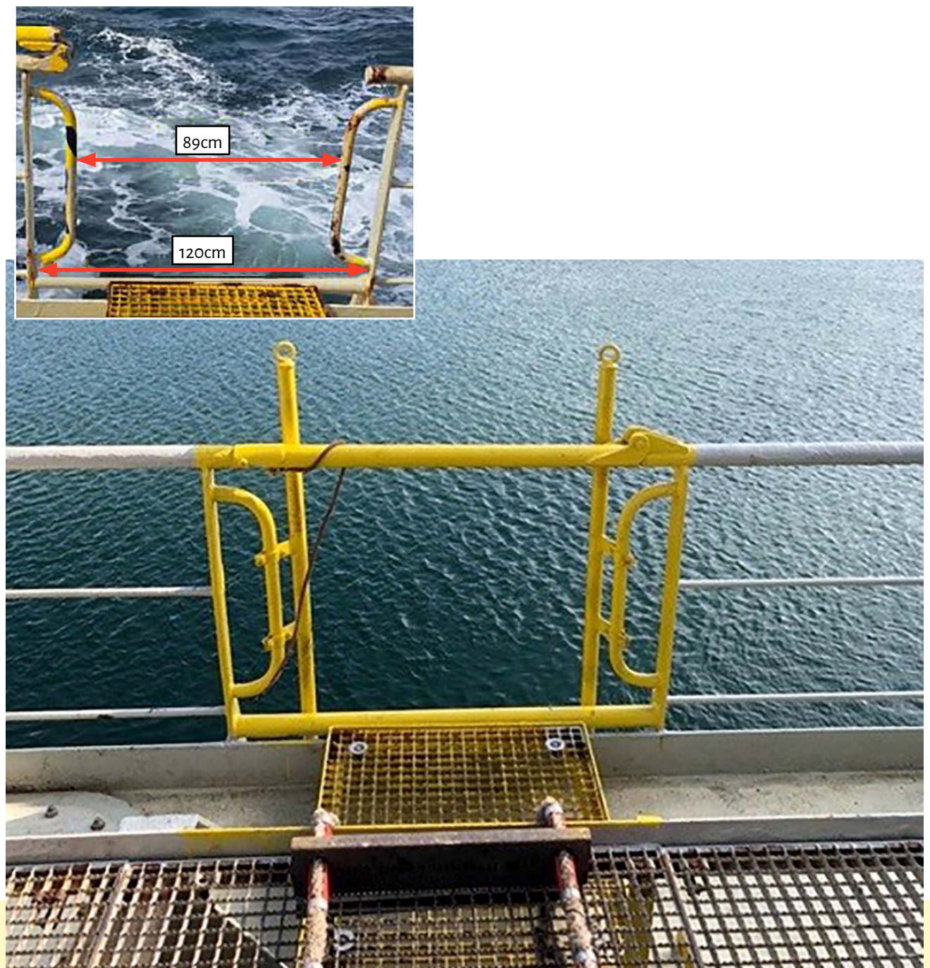
Figure 2: Guard rail gate at the top of the pilot ladder before (inset) and after modification to make it compliant
