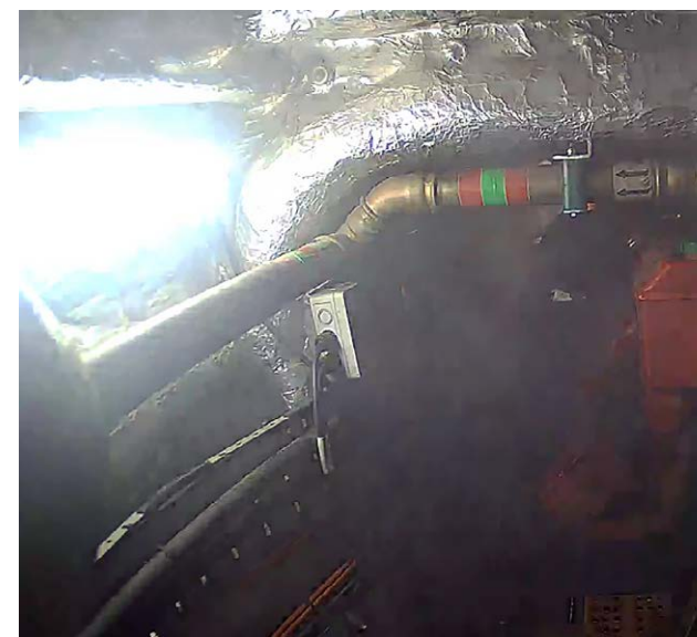
Figure 1: CCTV still showing smoke in engine space
