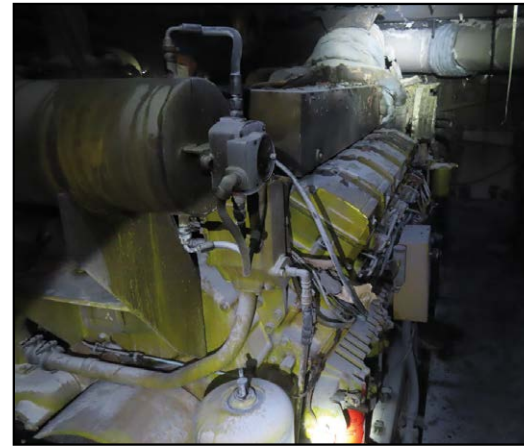
Figure 1: Damage sustained to auxiliary engine room
